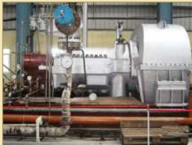
27MW Cogeneration Steam Turbine (Double Controlled Extractions) under Mechanical Run Test
